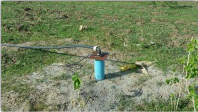
Bore hole water source
